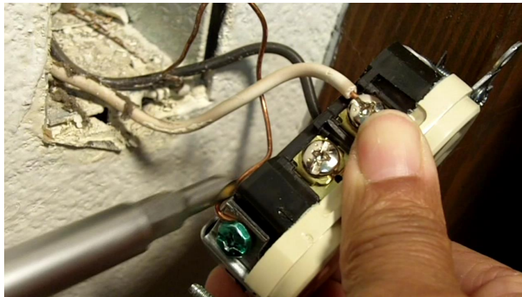
Ground and neutral on the existing outlet
